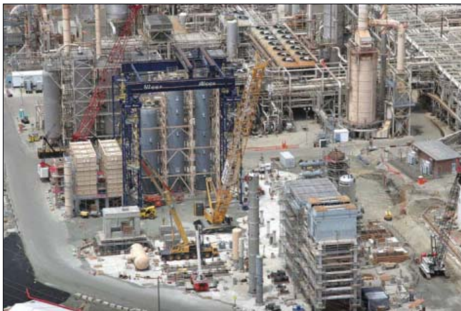
ConocoPhillips is constructing a 20,000-b/d hydrocracker at its Rodeo, Calif., refinery. Photo from Bigge Crane & Rigging Co.
