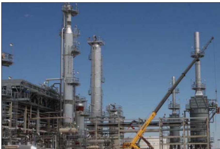
Work continues on Navajo Refining Co.'s 15,000-b/d mild hydrocracker project in Artesia, NM. Completion is scheduled for December. KP Engineering is providing engineering, procurement, and construction services for the project. Photo from KP Engineering.
