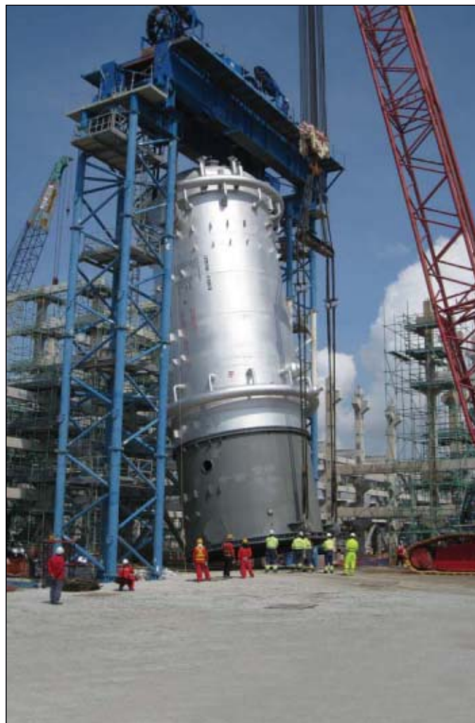
Workers install one of the two 1,375-ton reactors for the world-scale ethylene oxide/monoethylene glycol plant at the Shell Eastern Petrochemicals Complex in Singapore. Foster Wheeler is involved in the engineering, procurement, and construction of the project. Photo from Foster Wheeler/Shell.
